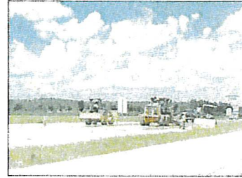
Crews work to complete the widening of the Foley Beach Express. Work to finish the widening of the highway is one of the capital projects on the Foley budget for the upcoming fiscal year.
