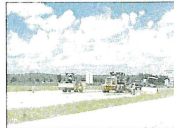
PHOTO: REPT/ALBC, GULFCOASTMEDIA.COM Crews work to complete the widening of the Foley Beach Express. Work to finish the widening of the highway is one of the capital projects on the Foley budget for the upcoming fiscal year.
