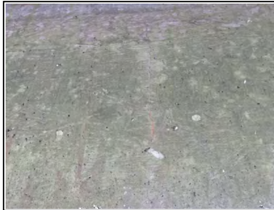
cracks span 10 girder 3
