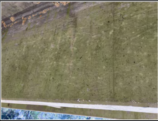
cracks in girder 3 span 10
