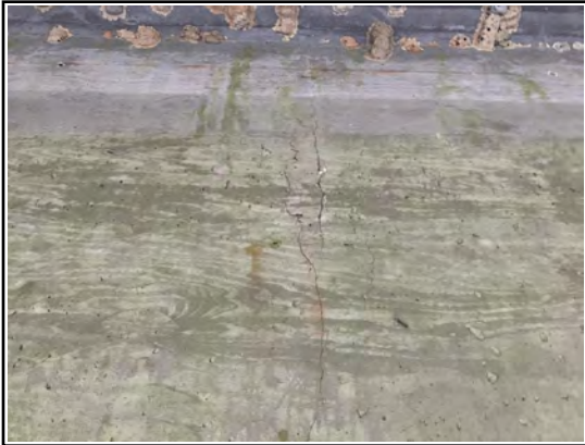
delam girder 2 span 11 left face
