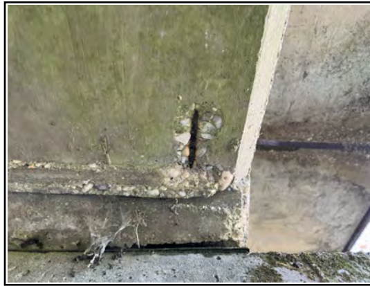
exposed rebar span 6 beam 1
