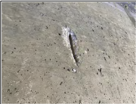
spall girder 2 span 11 right face
