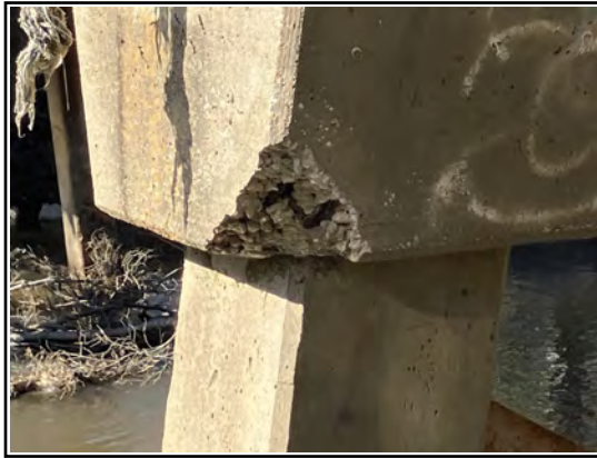
spall bent cap 11 right side
