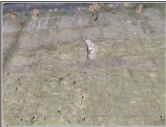
delam girder 2 span 11 left face
