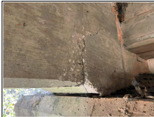
delam span 13 girder 3
