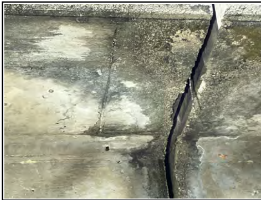
delam right overhang at bent 10 span 9
