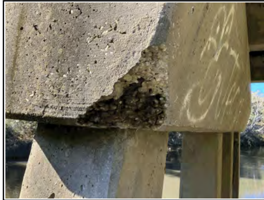
spall bent 11 cap right side
