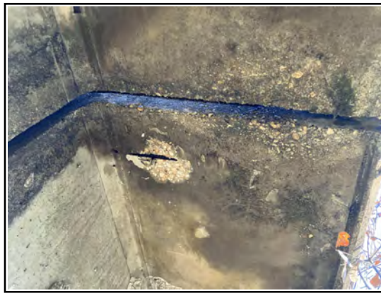
spall right overhang at bent 4
