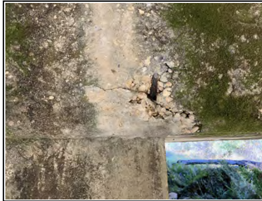
spall bent 3 cap over pile 2 far face
