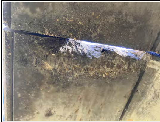
spall left overhang at bent 13
