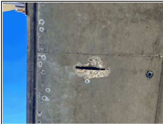
spall right overhang span 5
