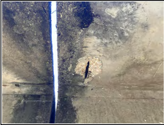
spall span 4 right overhang at bent 4
