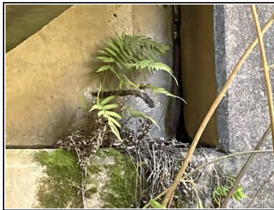
exposed rebar abut 1 near beam 1
