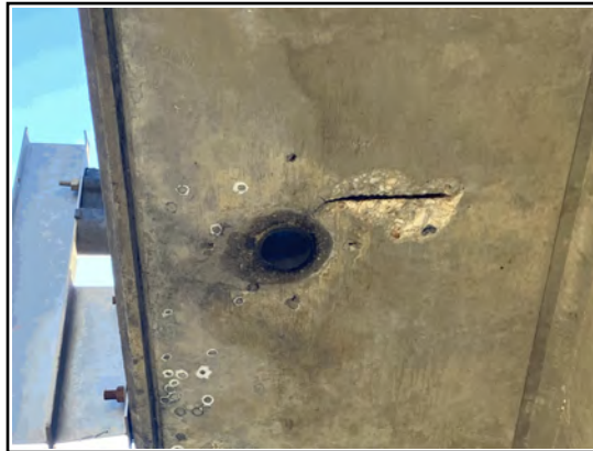
spall right overhang span 5
