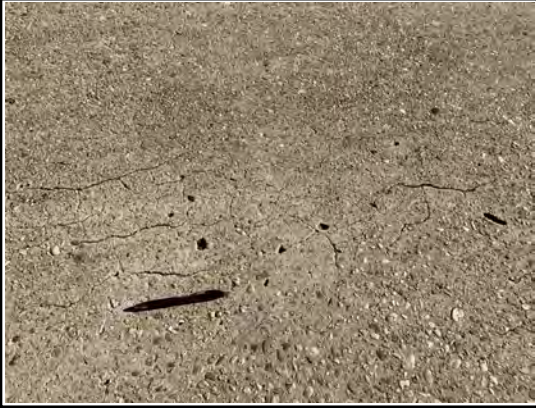
deck map cracks span 2
