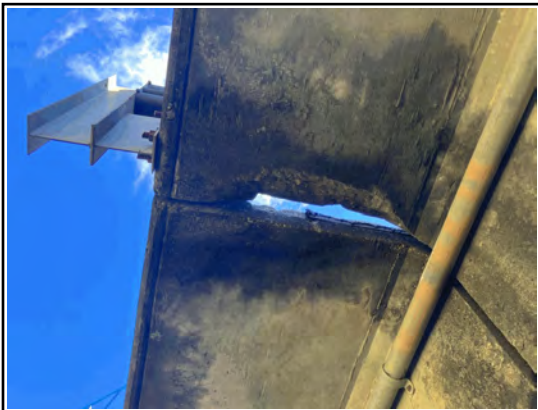
spall span 3 left overhang at bent 4
