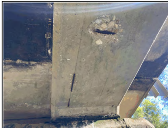
exposed rebar girder 3 at bent 7
