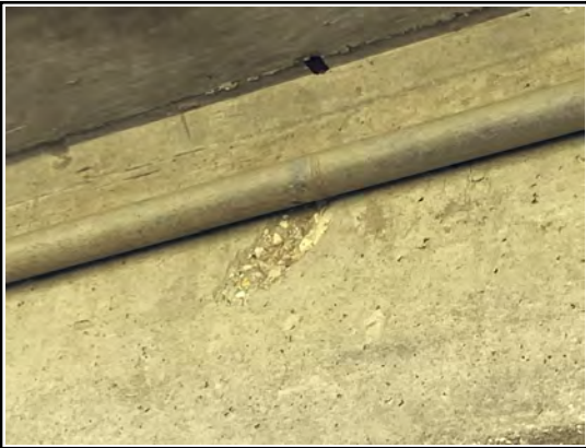
spall span 4 outside beam 1
