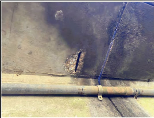
spall left overhang at bent 3
