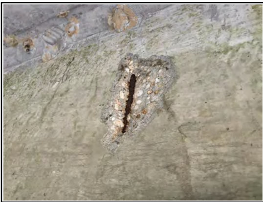
spall span 4 girder 2 left face
