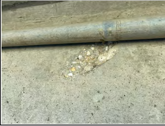
spall span 4 outside of girder 1
