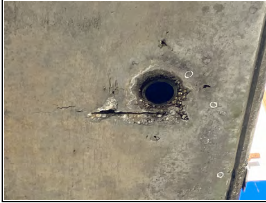
spall right overhang span 5
