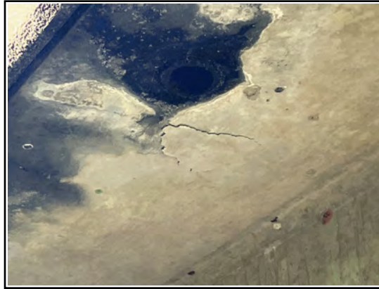
delam span 4 right overhang
