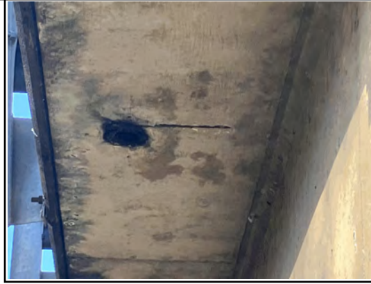
spall span 6 right overhang
