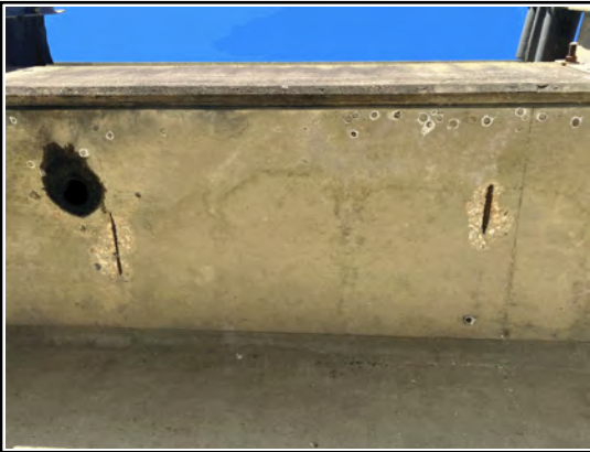
spalls span 4 right overhang
