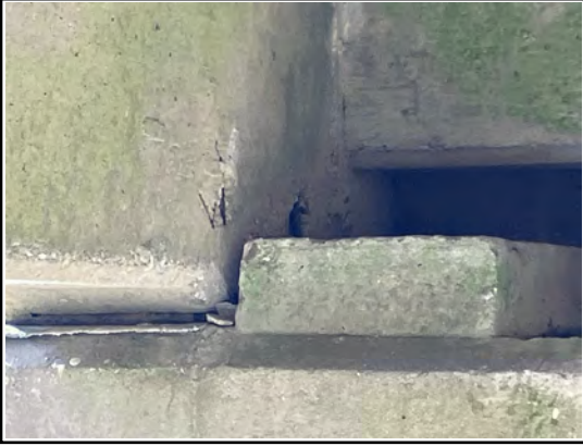
spall inside beam 3 at bent 6
