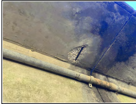
spall span 3 left overhang at bent 3
