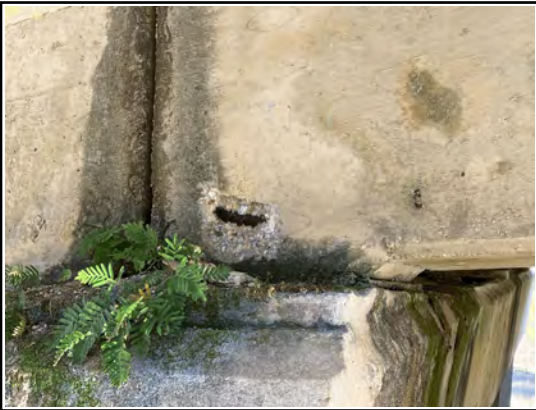
spall beam 1 at bent 9
