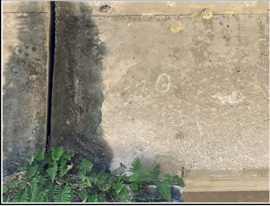
shear crack beam 1 at bent 10
