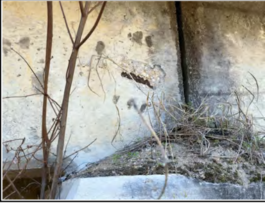
spall beam 3 at bent 9
