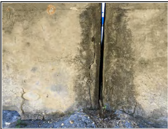
vertical crack beam 1 at bent 2
