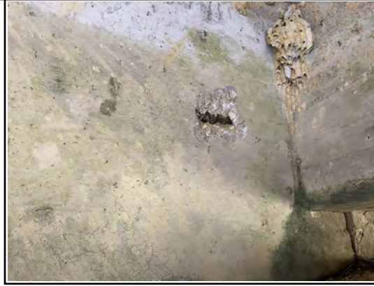
spall beam 2 at bent 9
