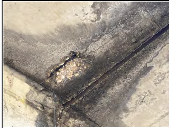
spall right overhang at bent 10
