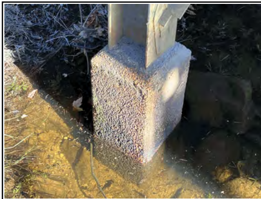
abrasion on piles
