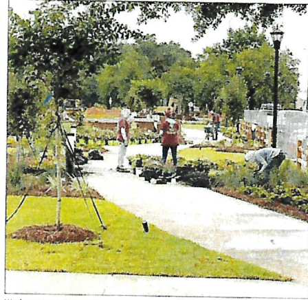
Workers are completing the green space next to the post office in Foley. The one-block project will link the two sections of the Perry Wilbourne Rose Trail.
