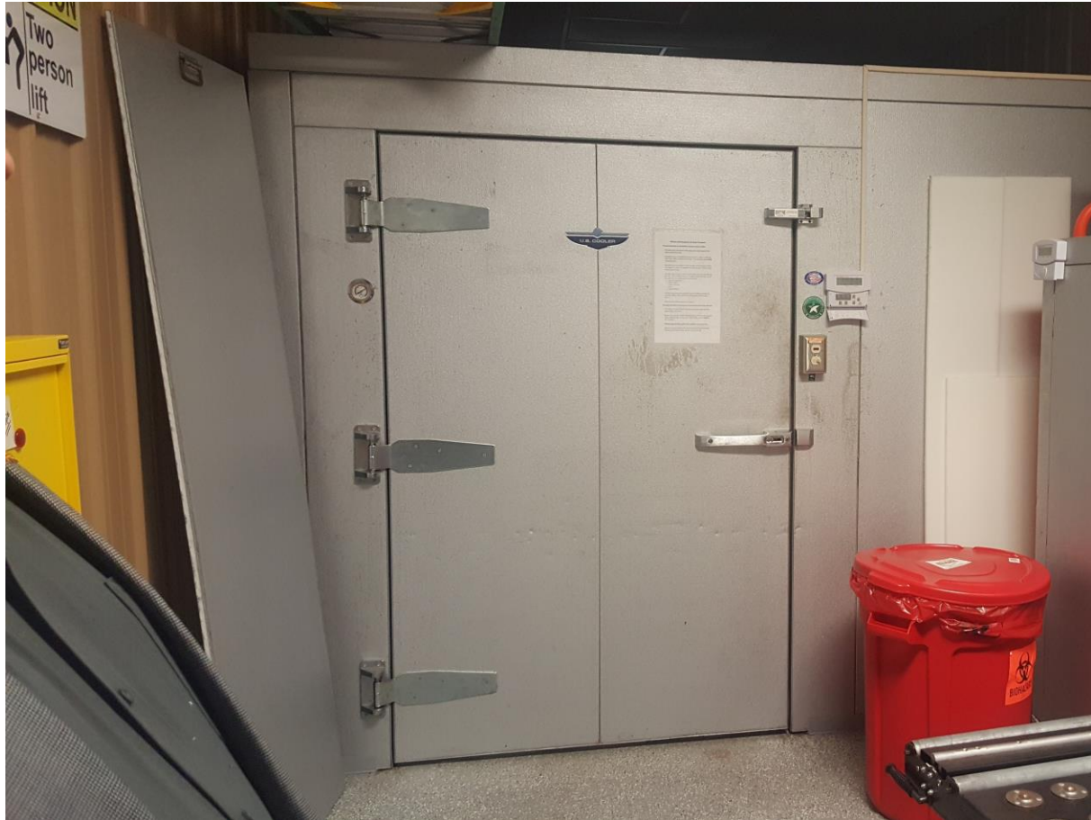
Decedent Cooler unit in the cooler area
