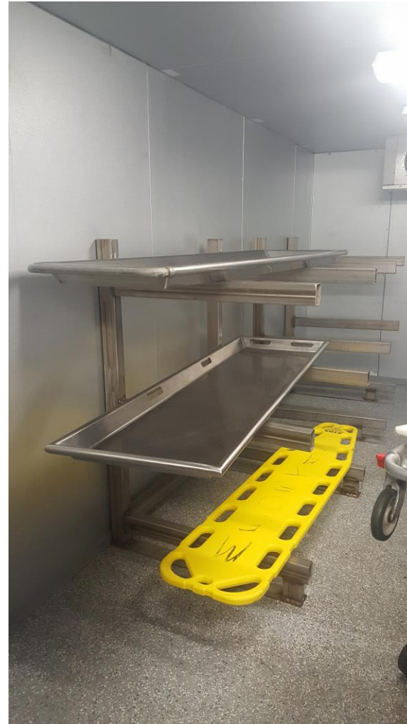
Inside view of the Cooler Unit
